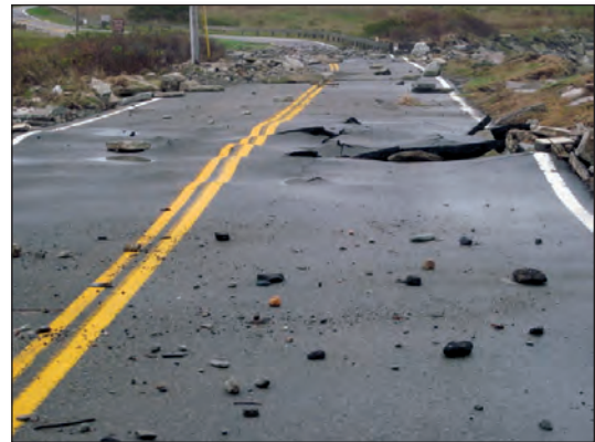
Hurricane Sandy damage at Sachuest Point National Wildlife Refuge.
