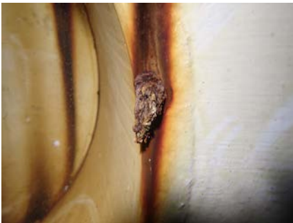
Interior Manway #1 Photo of metal exposure
