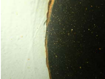
Interior Manway #2 Photo of metal exposure
