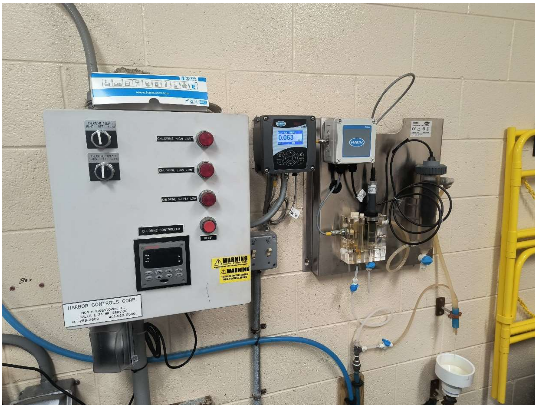
8: Limerock Pump Station Chlorination System
