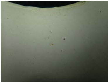
Interior Manway #1 Photo of corrosion
