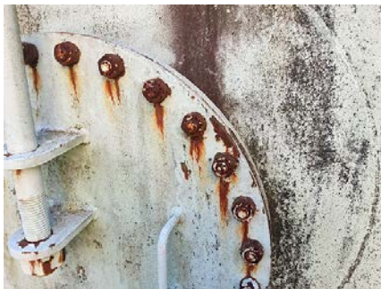
Photo of corrosion
