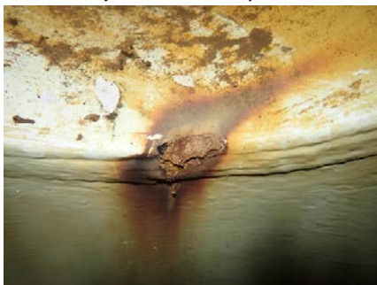
Interior Manway #2 Photo of metal exposure
