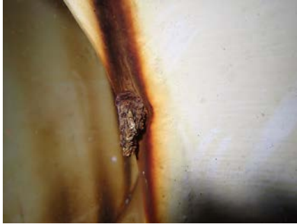
Interior Manway #1 Photo of corrosion
