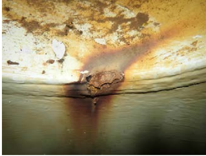
Interior Manway #2 Photo of corrosion
