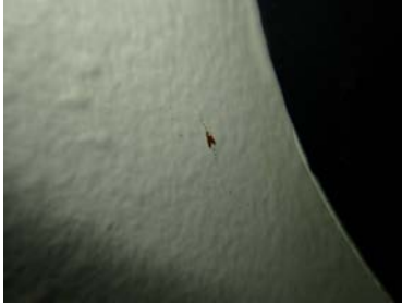
Interior Manway #1 Photo of metal exposure
