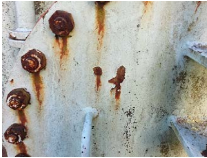
Photo of metal exposure
