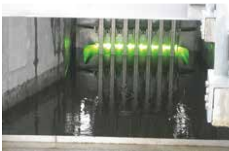
Ultraviolet disinfection system at Easton’s First Beach (City of Newport)
